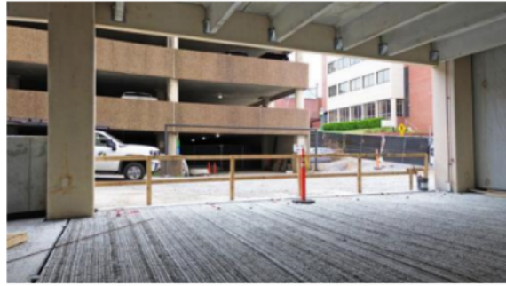
Secured Entrance to CC1SPG at Commerce.
